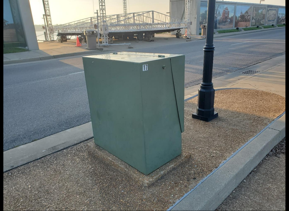
East electrical switchbox
