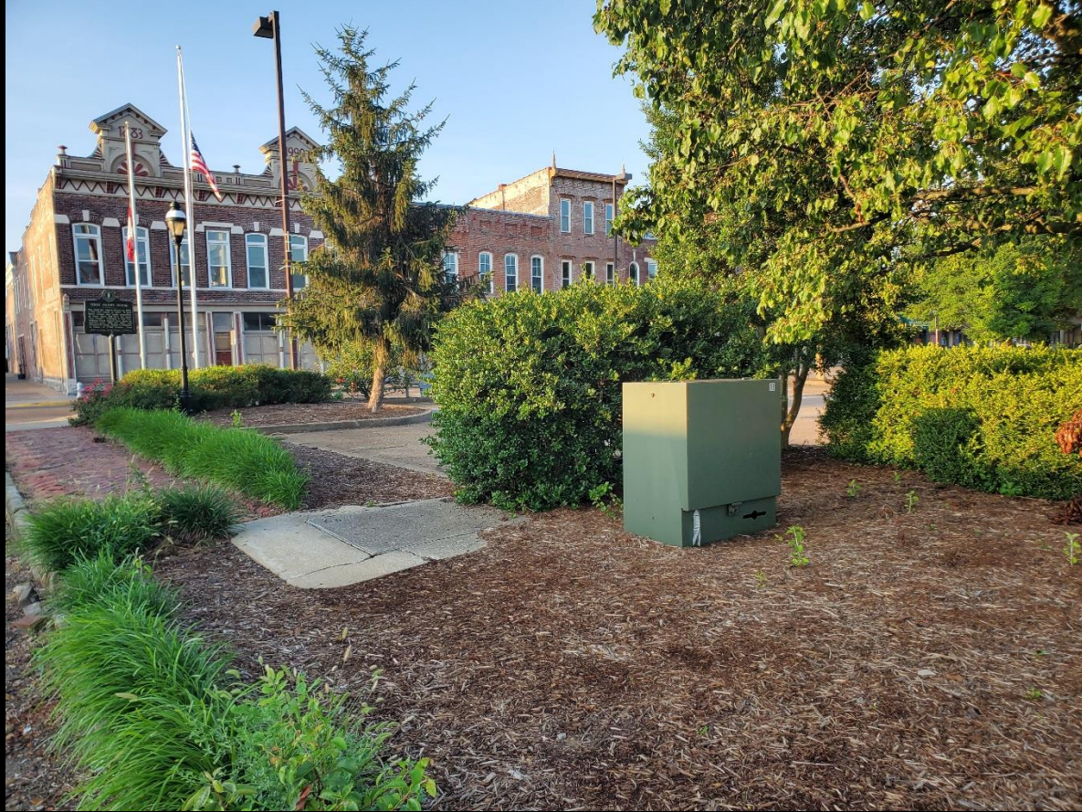
SE corner electrical switchbox
