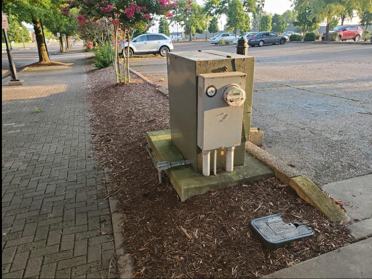
SW corner electrical switchbox
